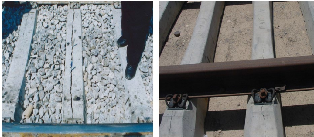
Fig. 2. Longitudinal cracks of the B70 type sleeper during operation (left) and new sleepers (right), (Source [2]).
