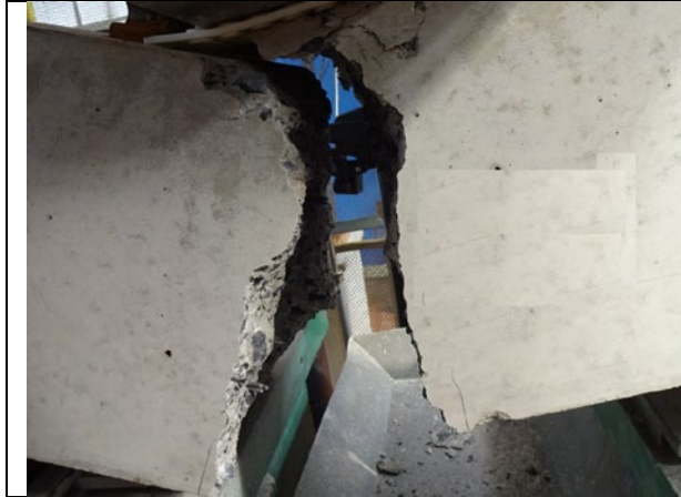
Fig. 7. Fracture of the PS-94 sleeper reinforced with a braided wire.
