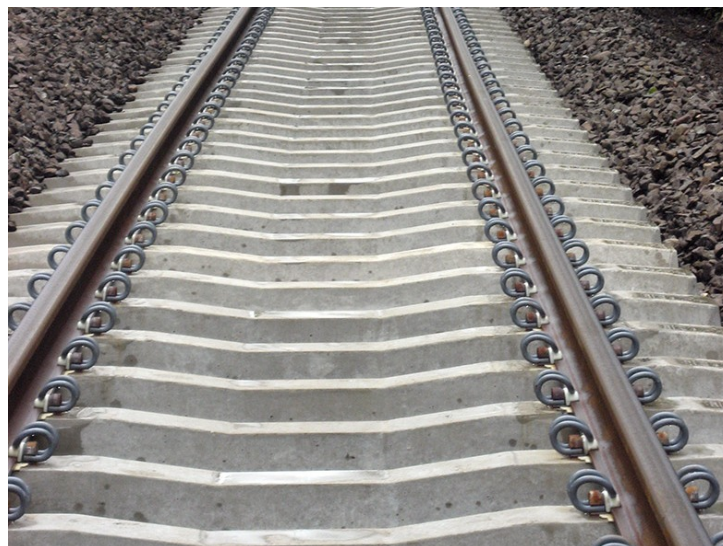
Fig. 12. A section of the rail road with sleepers that have reinforcement with braided prestressing wires (source: [5])
