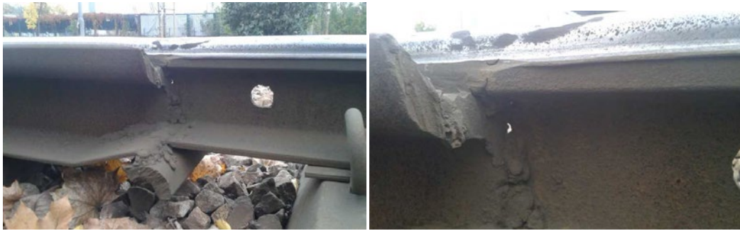
Fig. 2 Low quality of the rail joints – clearance, lack of material under rail head.
