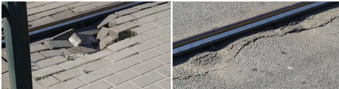
Fig. 3 Low quality of the tram tracks maintenance.
