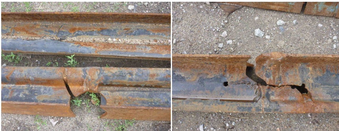
Fig. 4 Crack of the rail in the area of the rails joint.
