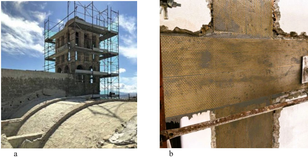
Fig. 25 (a,b) . Application of FRCM on vaults: a. [41], b. PBO and carbon long fiber reinforcement FRCM on reduced section concrete structures (such as floor joists) with 105 g/m 2 unidirectional PBO mesh and MX-PBO Concrete inorganic matrix. [42]
