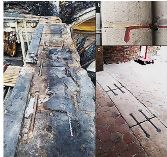
Fig.9. Notre Dame Cathedral, Paris. Detail of iron staples: a. south nave, b. monolithic columns nave, c. choir stand.[18]
