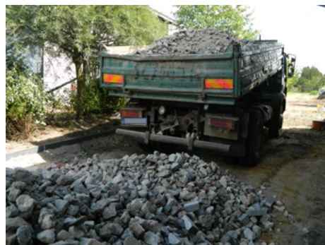
Fig. 1. The use of crushed concrete in the construction of the pavement base (photo: Z. Respondek)
