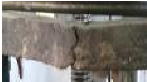
Fig. 5 Photographic View of Slab Failure
